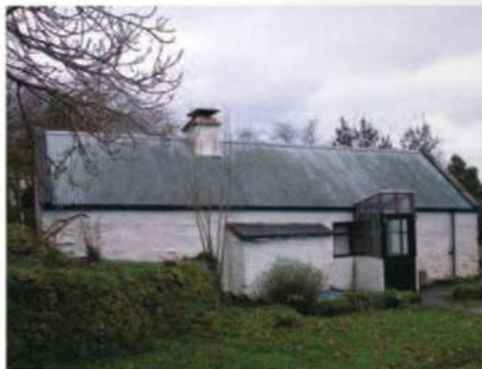
The 'unique' design of porch with the result being no windows to the front (west elevation).
